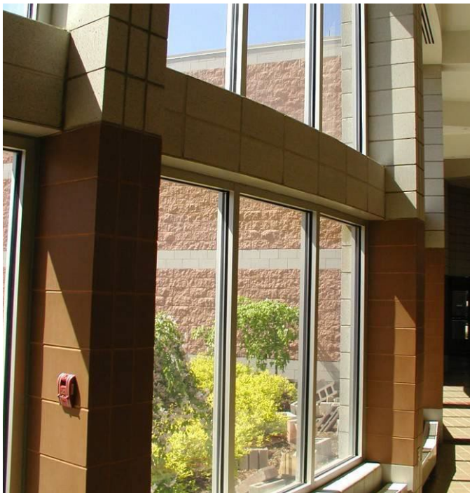
Concrete block between upper and lower windows allowing water infiltration – flashing is suspect.
