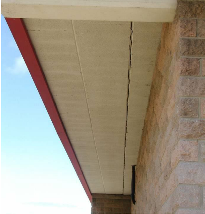
Concrete plank roof shifting at Besser Technology Center – connecting cables are suspect.
